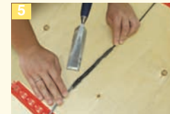
Make a groove to hold the cold lead connection with the heating cable.
