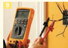
When connecting the system to the thermostat, test the integrity of the cable and record the readings on the measurement table.
