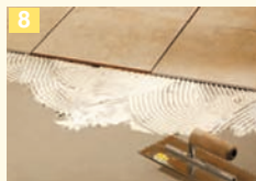
Spread self-levelling cement and allow to dry. Floor covering may now be installed. Test the integrity of the cable before and after embedding the heating cable in cement and record the readings on the measurement table.
